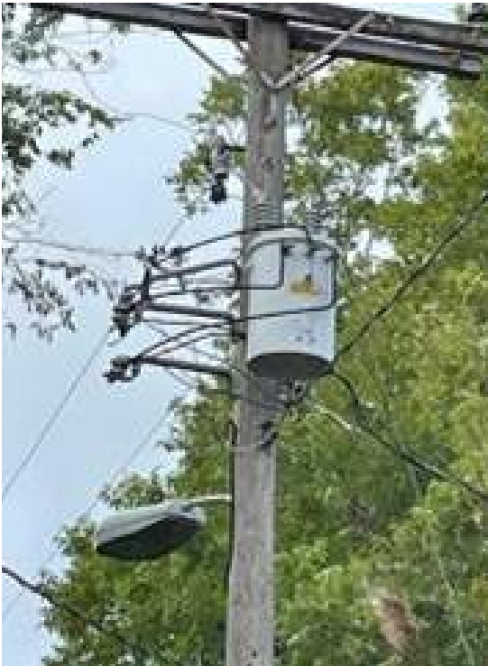
Electric Pole Beside Caretaker's Cottage
