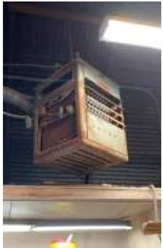
Equipment for the Quonset Hut
