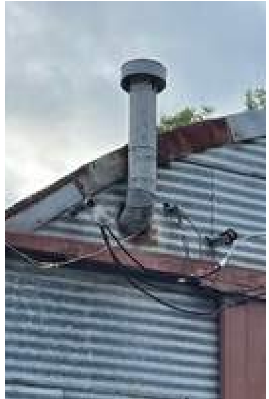
Ventilation of Quonset Hut
