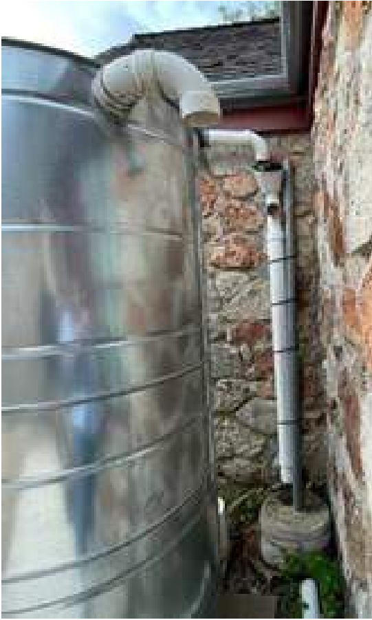
Rainwater Treatment of Caretaker's Cottage
