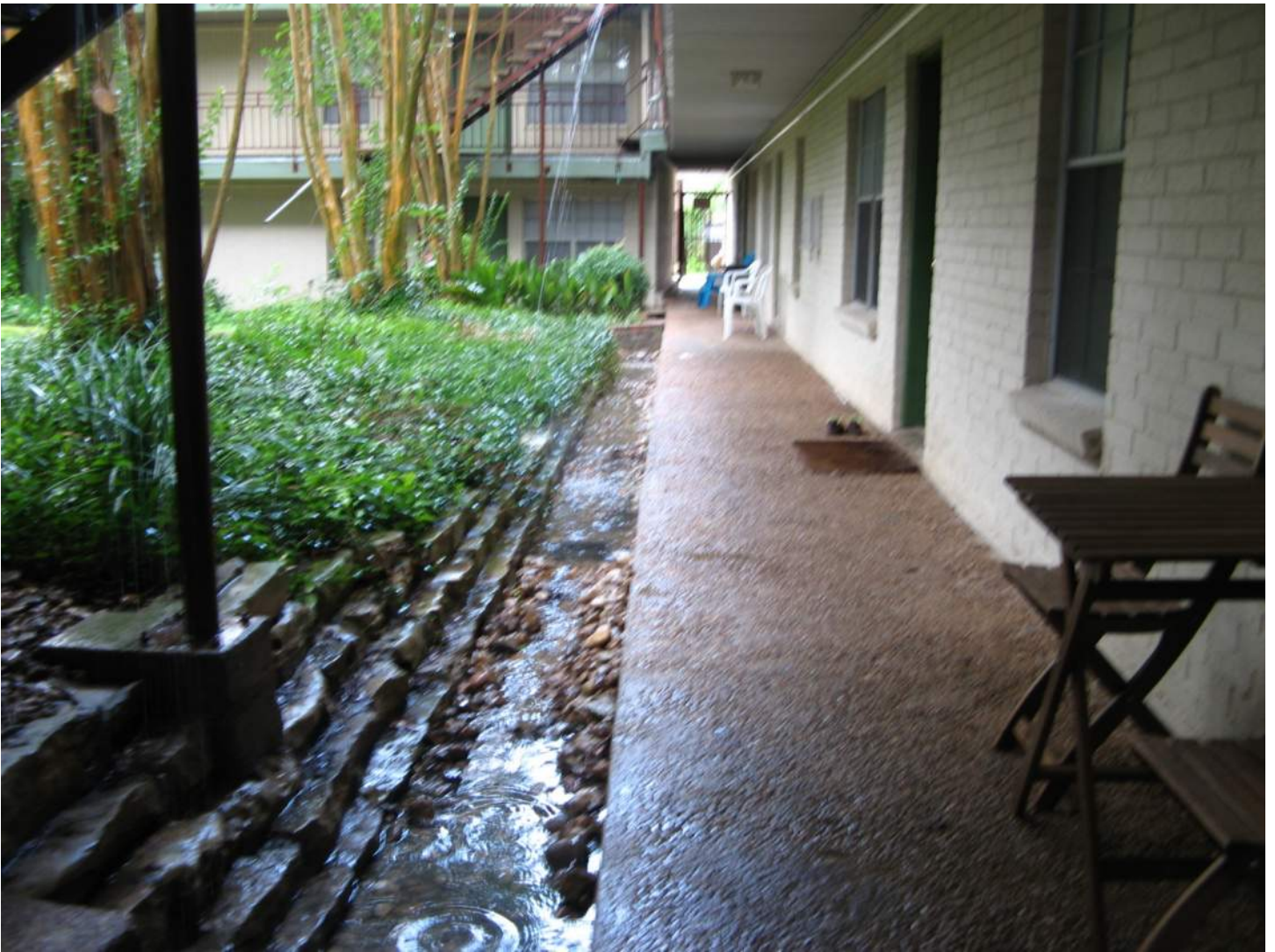
View from northeast corner of interior courtyard – units on the right side of photo flood
